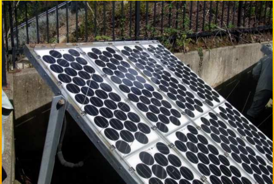
29 years old silicone laminated PV panels (Japan)
